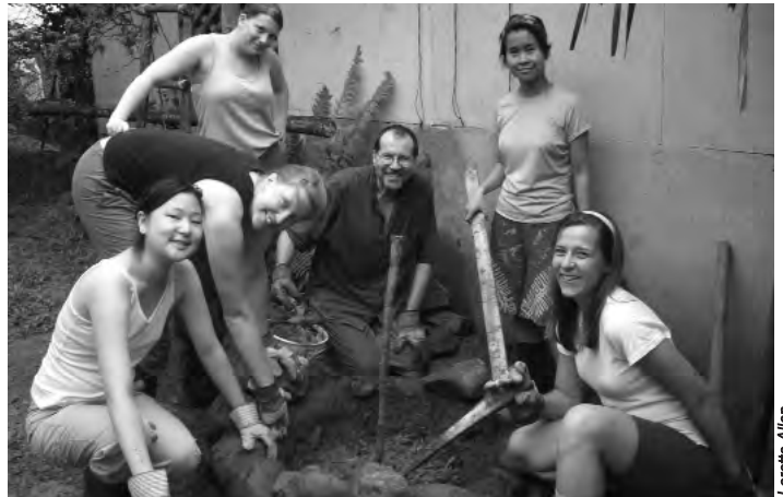
Centre for Environment students in Costa Rica making a foundation for a cob oven (made of mud, sand, and straw), one of the activities of their work placement in the Professional Experience course. David Powell, work placement coordinator (centre), joins students, from left to right, Irme Chan, Dawn Strifler, Loretta Allen, Paw Wah and Elena Jusenislika.
